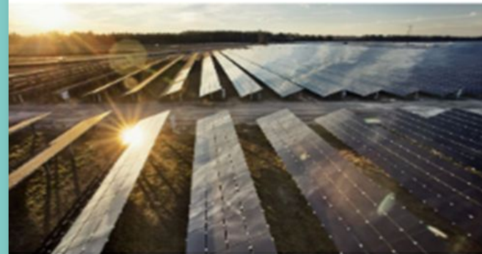
Sol Systems will build and operate 500 megawatts of solar as part of a new partnership with Microsoft. Credit: Sol Systems.
